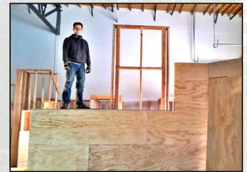
Jevin stands on top of work in progress structures for the gym.
